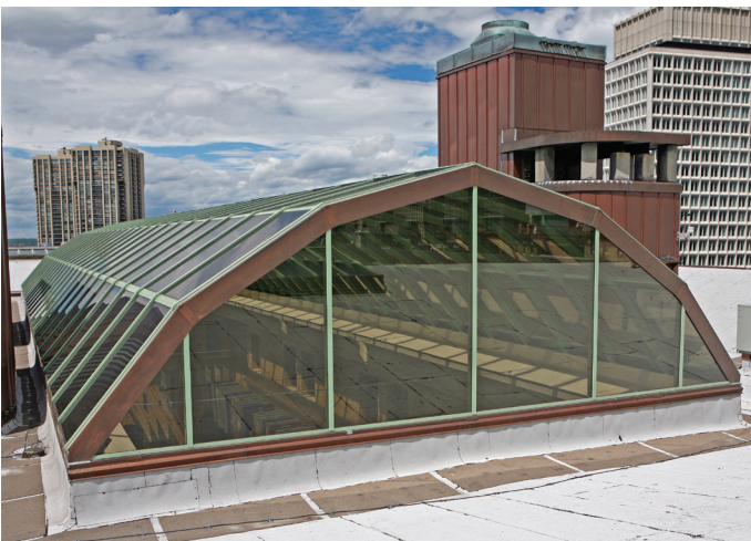
The large atrium skylight is a Pinnacle Segmented Vault with integrated OKALUX photovoltaics in the center.
