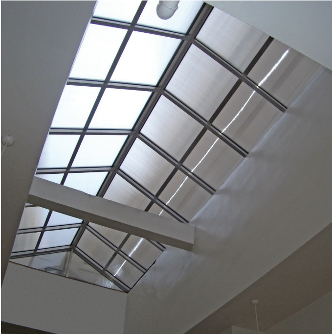
Large Horizon polycarbonate skylight system over the active kitchen area in the busy hotel restaurant.
